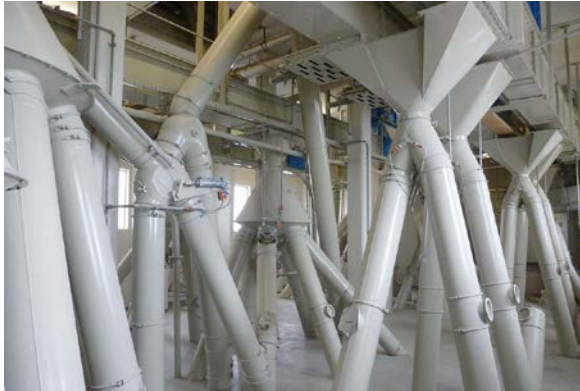
Figure 3: View of raw materials sorting system
